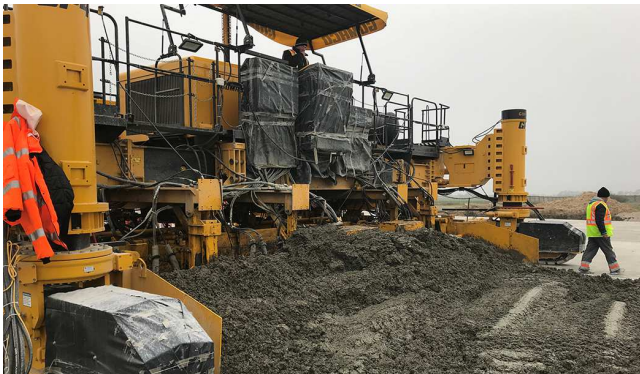
Picture 1: Concrete with MCE™ can be placed using traditional methods, including slipform paving.
