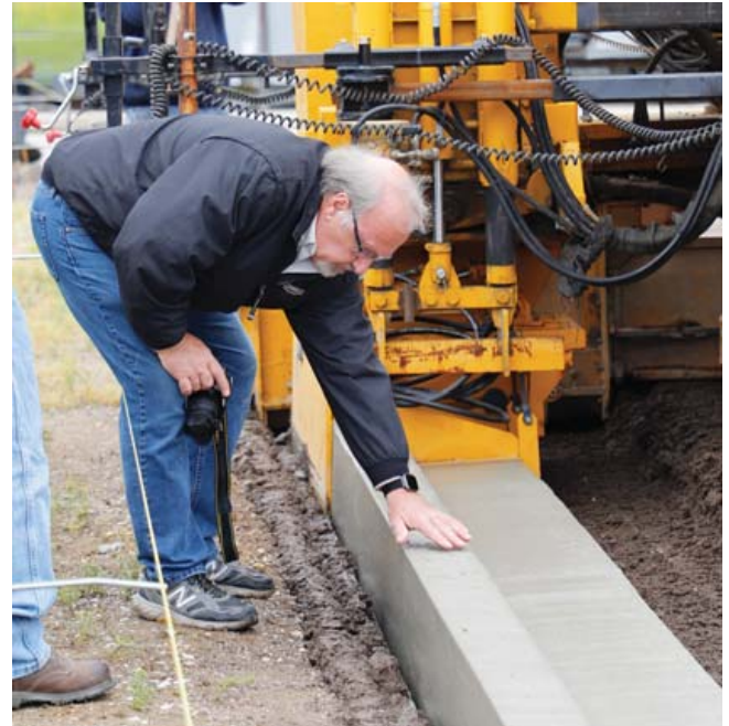
Picture 2: Dr. Mike Ayers inspects concrete curb and gutter with the MCE™ additive
